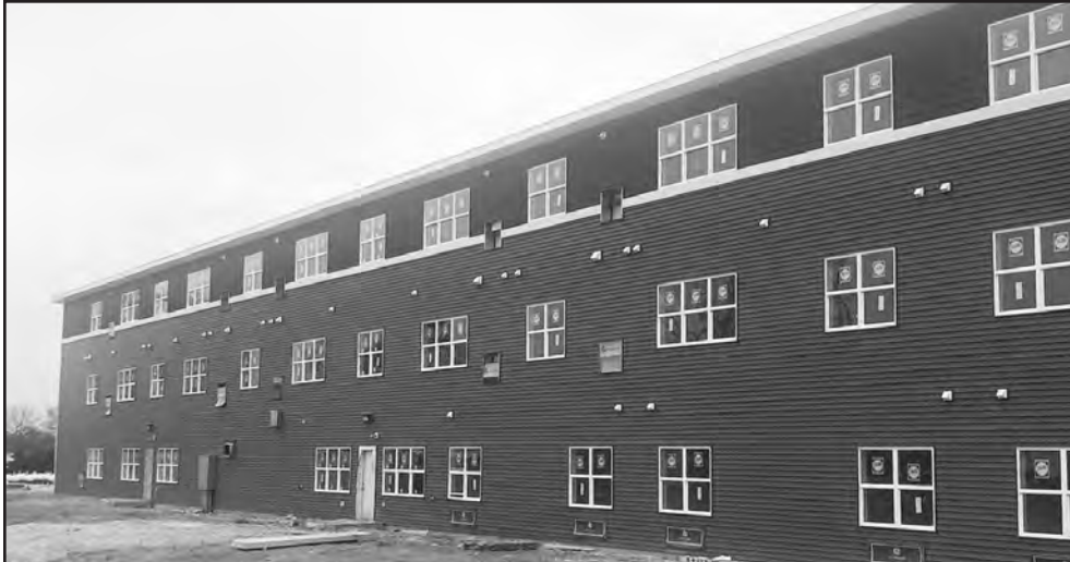
View of back of building. Here will be 2 patios with furniture for residents to enjoy. The Memory Care Patio will also include a walking path.
