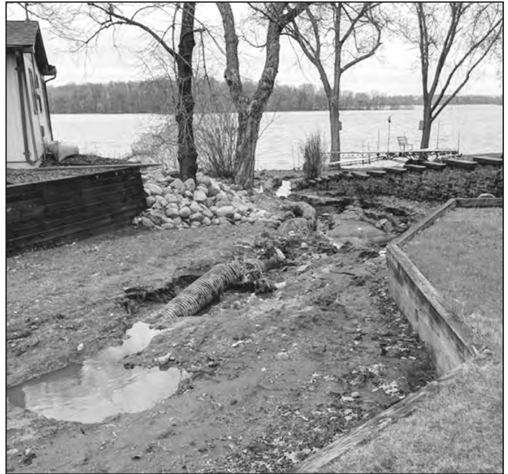
BEFORE: The worsening gully between neighboring properties on Circle Lake southeast of Lonsdale is shown on June 21, 2019. Landowners worked with Rice SWCD staff and Southeast SWCD Technical Support JPB staff on a solution. To fund the work, the SWCD used local capacity dollars — provided by Clean Water Funds from the Minnesota Board of Water & Soil Resources (BWSR) — and matching dollars from the landowners and the Circle Lake Improvement District.
