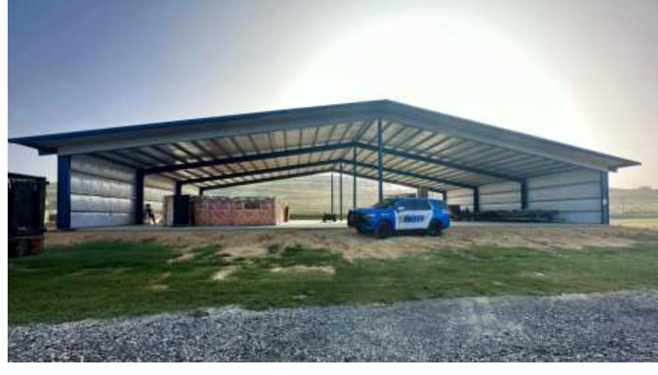
A custom metal building designed, manufactured, and installed by the team at Pipe & Steel. This project was commissioned by Livingston Parish Sheriff Jason Ard as part of the Sheriff's Training Center.
