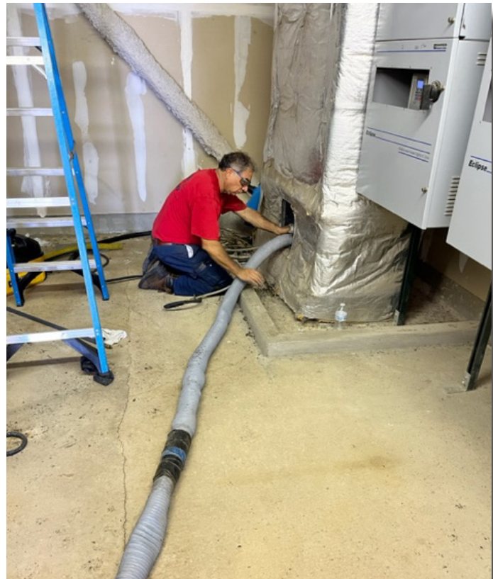
Steamatic employee Rene Salazar cleans ducts to remove mold and dust that trigger allergies; Steamatic is one of the few companies in the area that offers this service.
