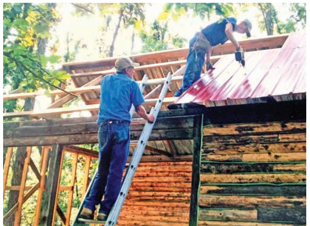
Ronnie Wilson gets a helping hand from his brother, Jimmy Wilson, putting the metal roof on the cabin. CONTRIBUTED PHOTO
