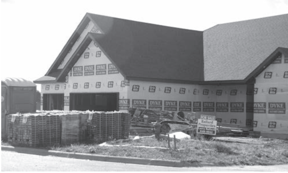
NEW HOUSES are under construction on East Ashford Avenue in Nixa, one of several places in northern and central Christian County where entire subdivisions are under development.
