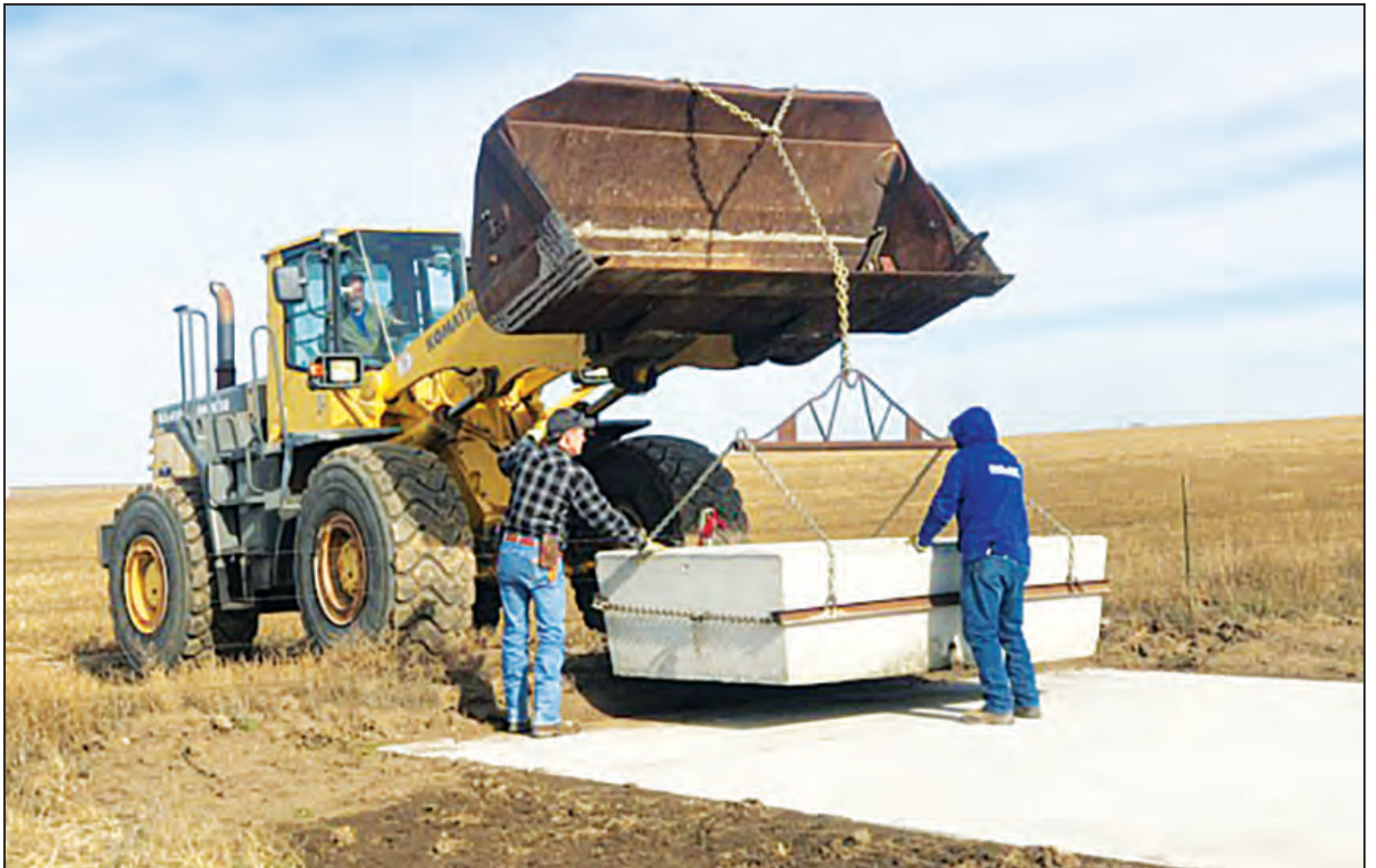
Erick Kadel drives, while Gabriel Lopez and Dustin Ole help set the rural water electric pump with pipeline laid a quarter of a mile to the pasture.
