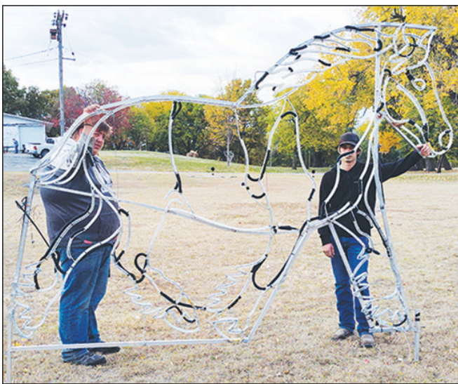
Heavy equipment and students from the Fort Hays Tech | North Central college put up the arches and the Diesel Department helped lay out the pieces at the Chautauqua Isle of Lights, soon to open on Wednesday, Nov. 27, the night before Thanksgiving.
