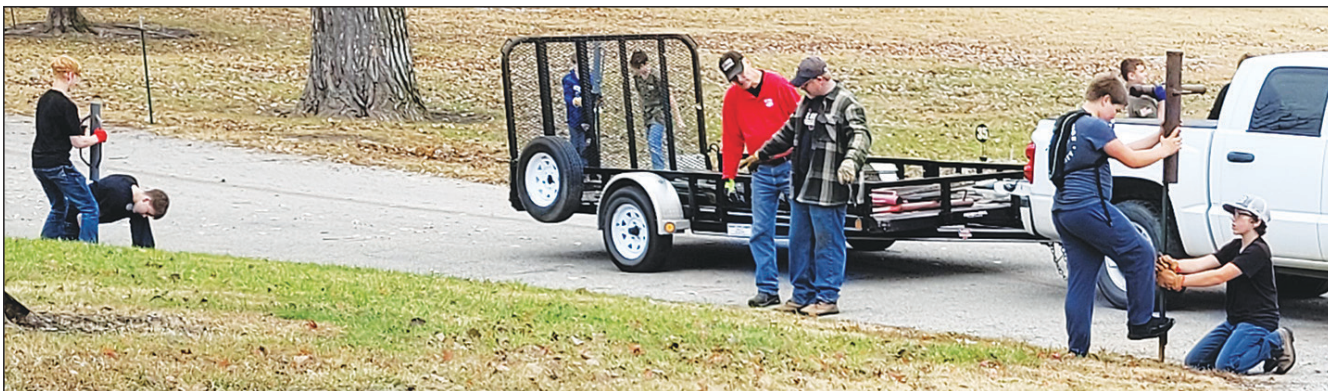
Beloit Jr. High students help put up steel posts that hold the road lights.
