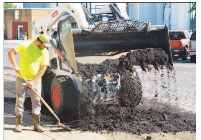
City of Beloit street crews have been keeping busy with resurfacing streets, including South Street.
